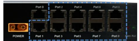
to Master Battery of each Group
